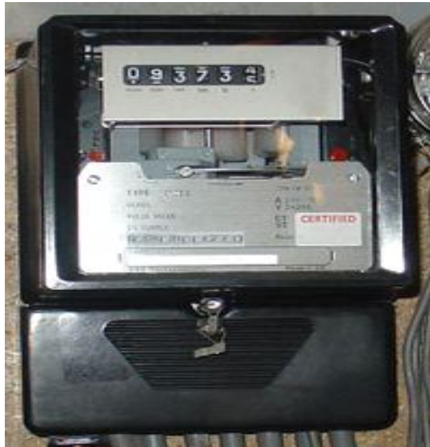
Fig 3.2 Three phase, Three wire energy meter
